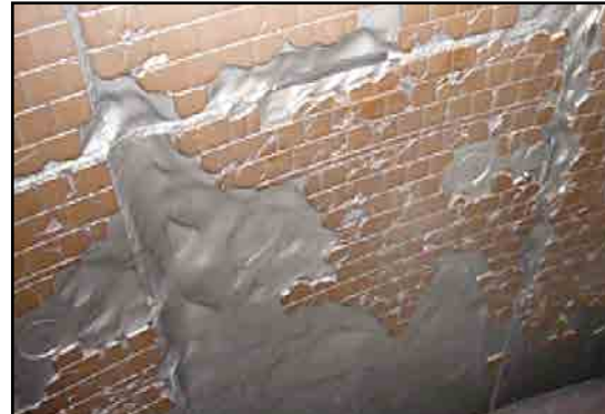
Damaged pulverizer walls
